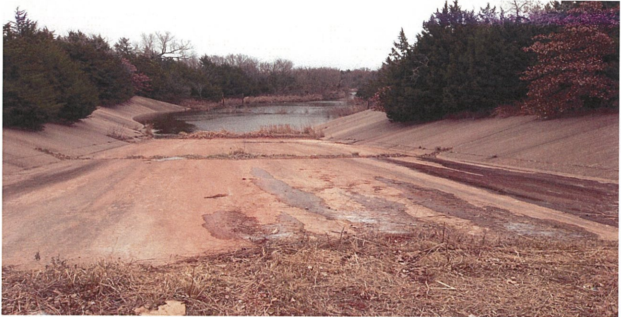
Figure 2827: Seepage through Joint on West Side of the West Spillway Channel
