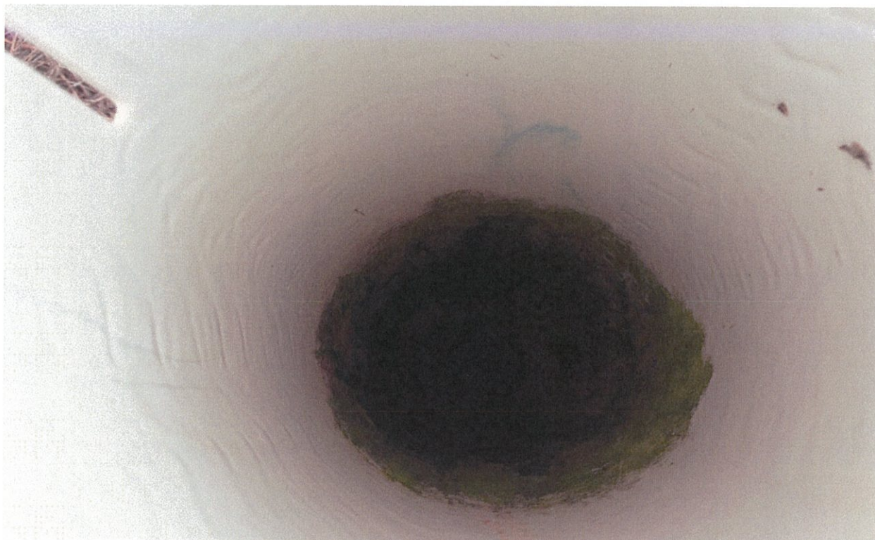
Figure 233: Water in Valve Riser
