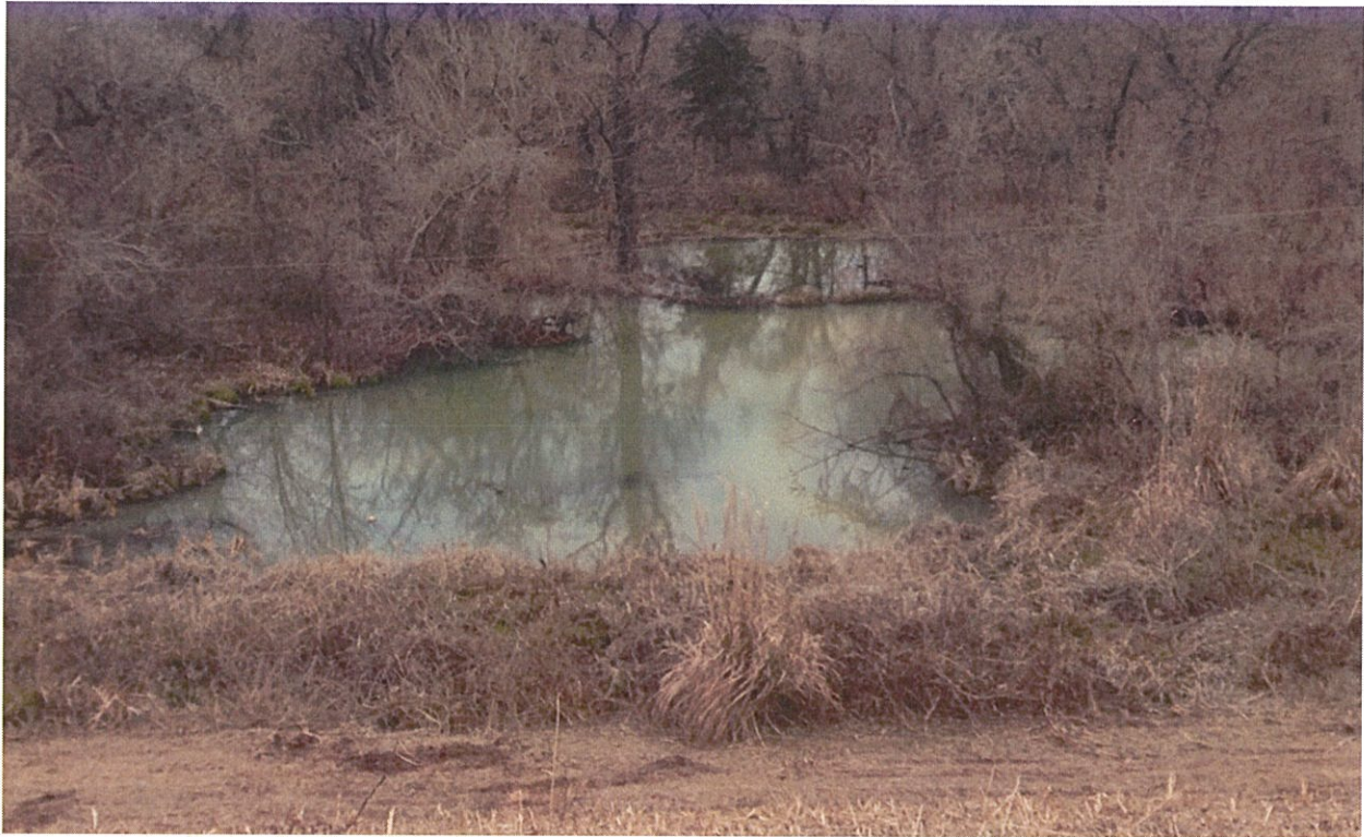
Figure 15: Standing Water at Toe of Dam – Photo Facing North from Crest
