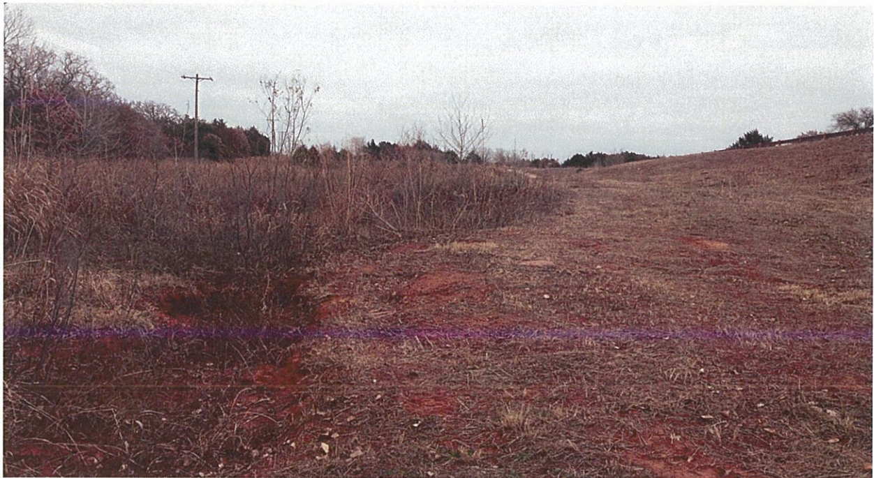
Figure 18: Erosion on East Abutment – Photo Facing East
