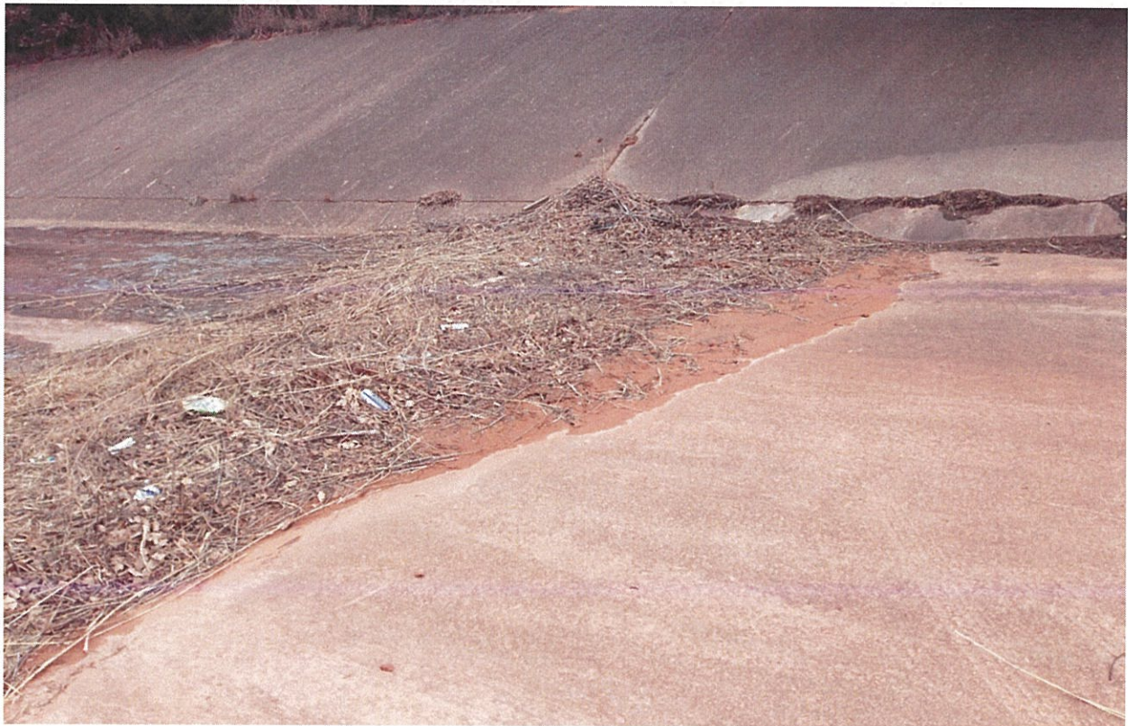
Figure 29: Seepage and Vegetation through Joints in West Spillway Channel
