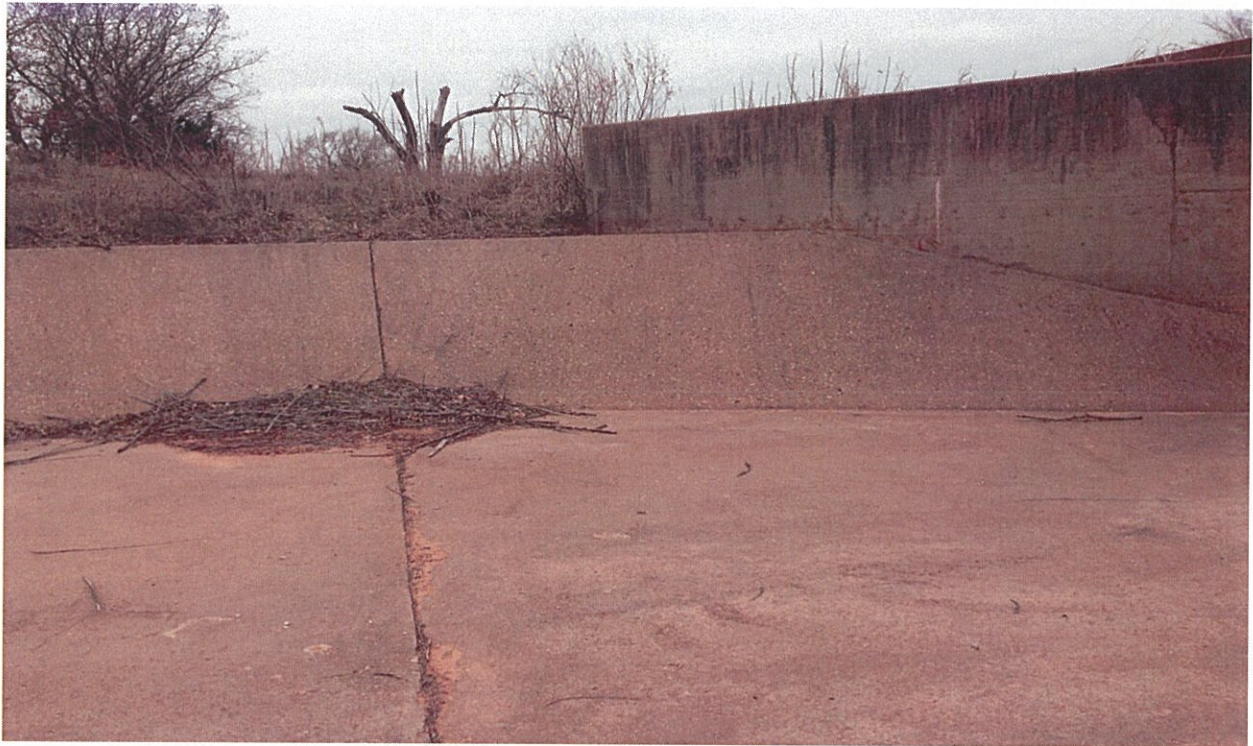
Figure 28: Spalling at Joint in West Spillway Channel
