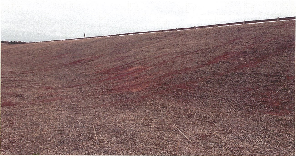
Figure 13: Inadequate Growth on Downstream Slope– Photo Facing SE
